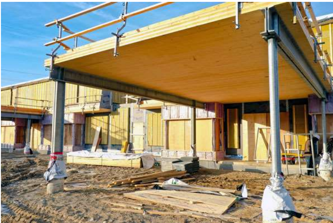
ELEMENT5 – The 781-square-metre building features cross-laminated timber (CLT) and glulam as the superstructure and cross laminated insulated panels as the envelope. Shown here is the CLT portico and outdoor play area.
