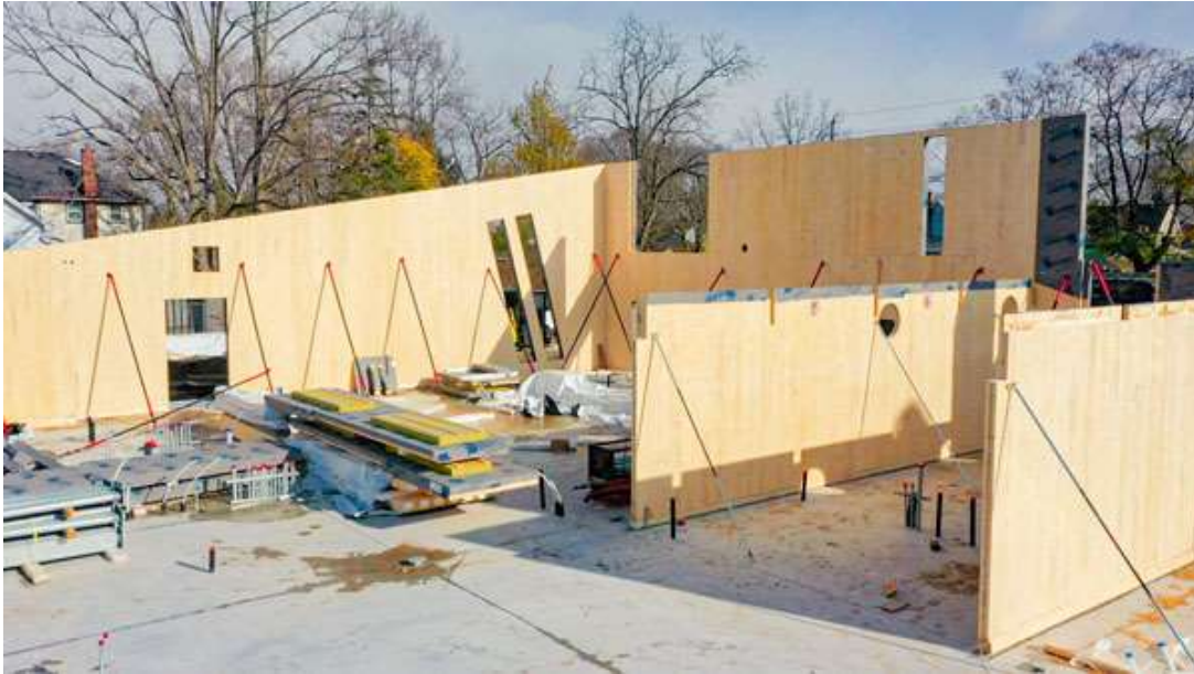
ELEMENT5 – Components of the child care facility included 1,005 square metres of cross-laminated timber (CLT) roofing, 535 square metres of CLT walls, 29 pieces of glulam columns, 43 pieces of glulam beams and 26 sections of steel columns.
