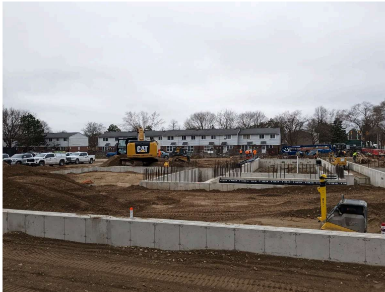
Ongoing construction at the site of phase one of the Reimagine Southdale project. Ben Harrietha/980 CFPL
